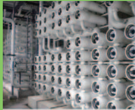
Waste Water Recycling Technology- RO Equipment
