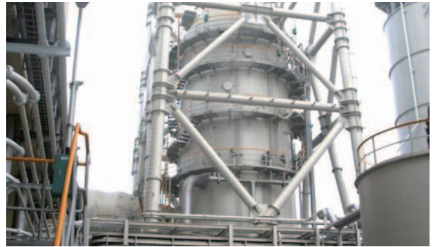
Flue-Gas Desulfurization (FGD) System
